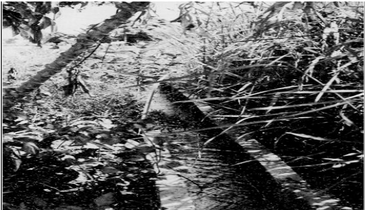
Figure 6: Heavy plant growth makes inspection difficult
